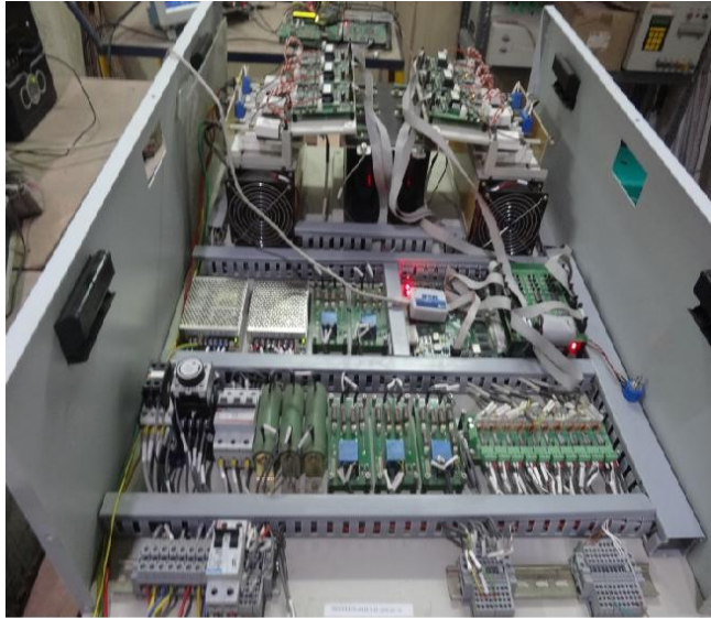
Fabricated converter- 10 kVA, FPGA based back to back converter
